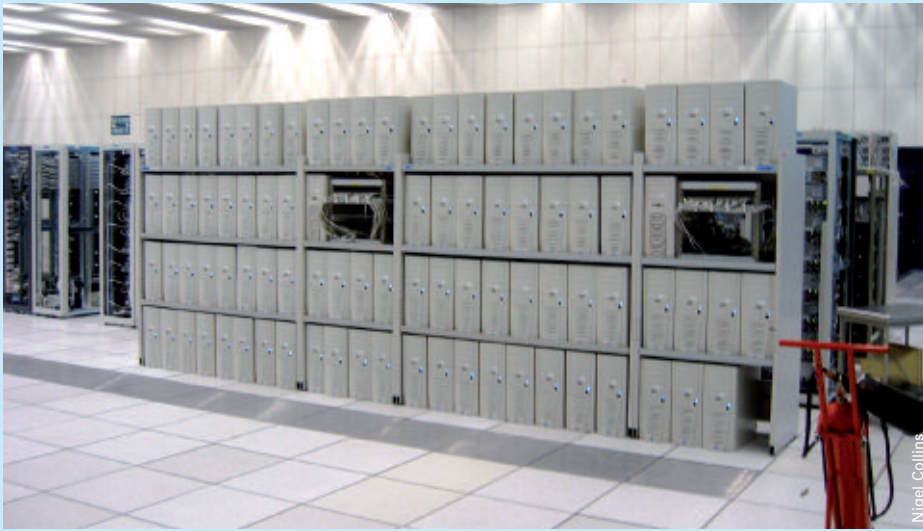
The computer hall at CERN with 2000 PCs per floor
