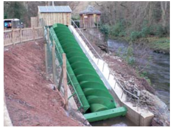
A micro-hydro system fully installed. This one is at Ashburton in Devon. The generator is in the wooden hut at the top.
