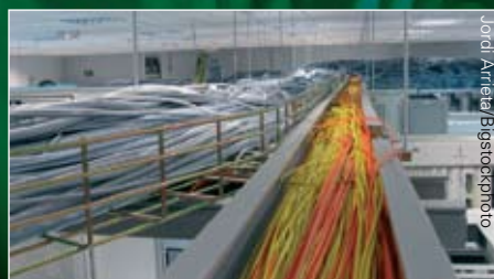
Electrical cables and optical fibres run side-by-side in a data handling centre.
