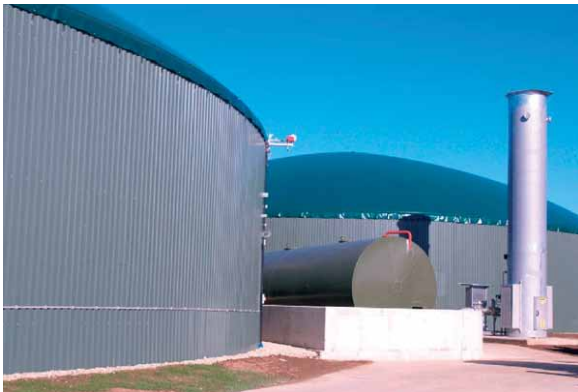
Two of the digesters at the anaerobic digestion plant
