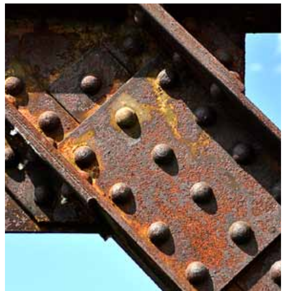
A complex metal joint, held together by rivets.
