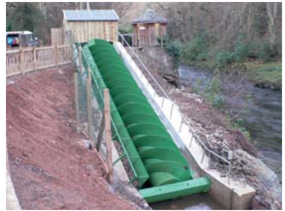
A micro-hydro system fully installed. This one is at Ashburton in Devon. The generator is in the wooden hut at the top.
