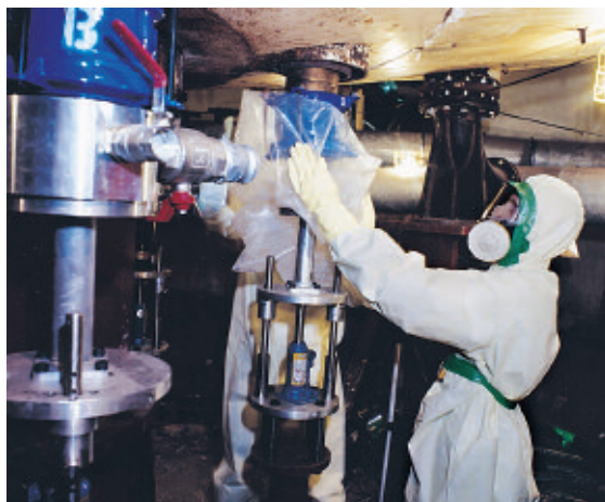
Workers underneath the main part of the Windscale advanced gas cooled reactor removing parts that might be contaminated
